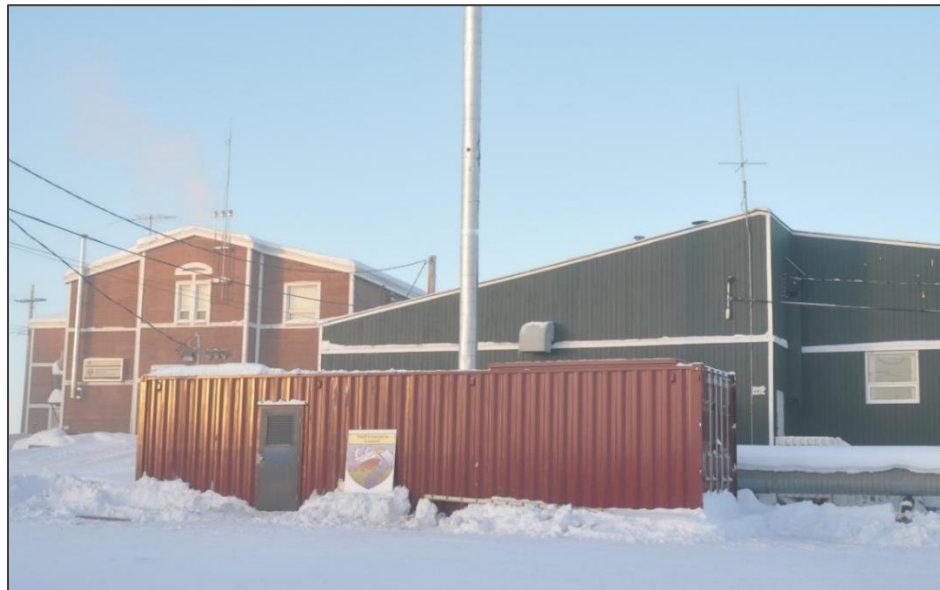
Figure 4: Fort McPherson biomass boiler, foreground, providing heat to the health centre and Band office in background (L. Keyte)
